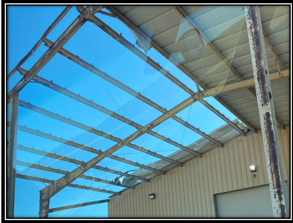
Photo No. 1 – Roof Damage from Hurricane
