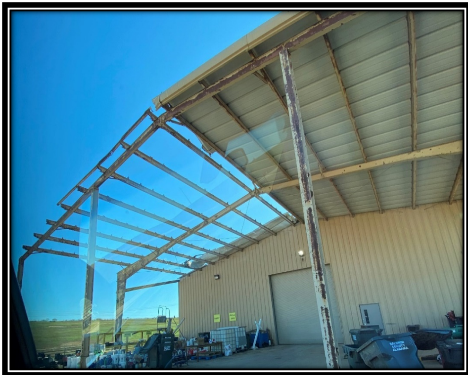
Photo No. 2 – Roof Damage from Hurricane
