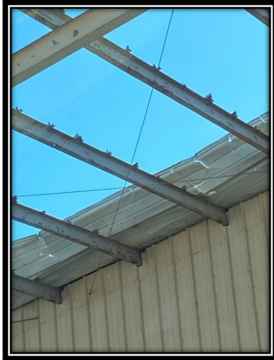
Photo No. 3 – Roof Damage from Hurricane
